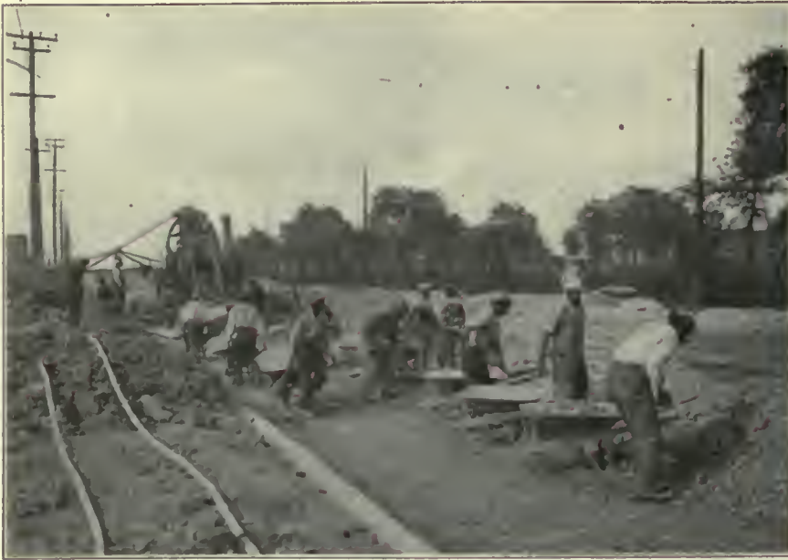
FIG. 49. STREET CONSTRUCTION, A SOURCE OF DUST. Street scene, September 1, 1914. Nearly 100 miles of streets are improved each year in Chicago. The handling of materials liberates large quantities of dust, which are borne by the wind over long distances.
